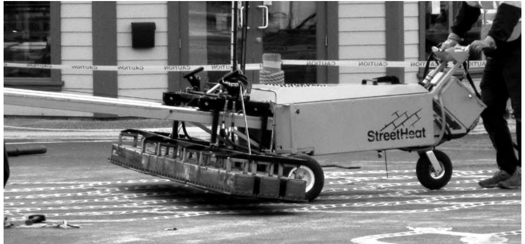
A worker uses a specialized infrared machine to install the artistic components of the new pedestrian scramble-style crosswalk at the intersection of No. 1 Road and Moncton Street. Photo: Christine Durgo
